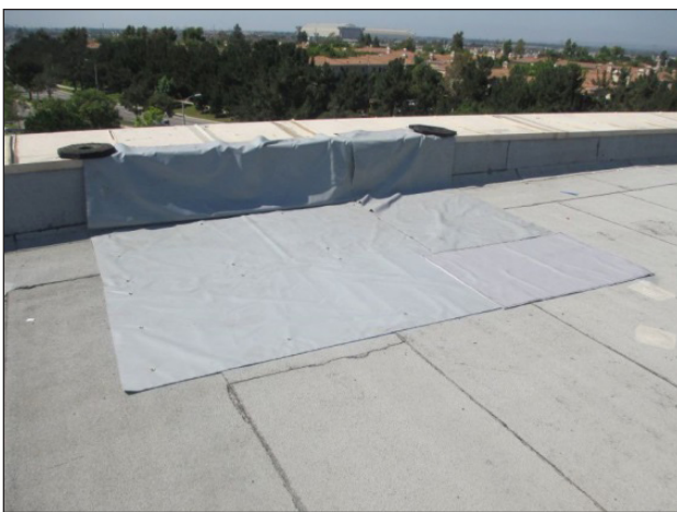
PIM Blankets deployed over large area generating PIM
